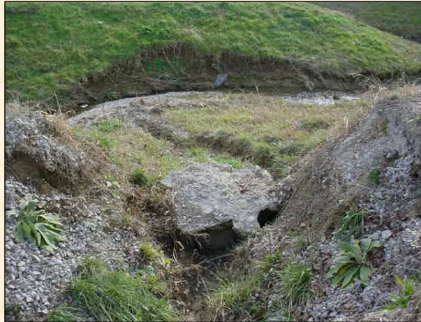
Figure 5 Severe Erosion Along East End of Sonntag-Stevens
